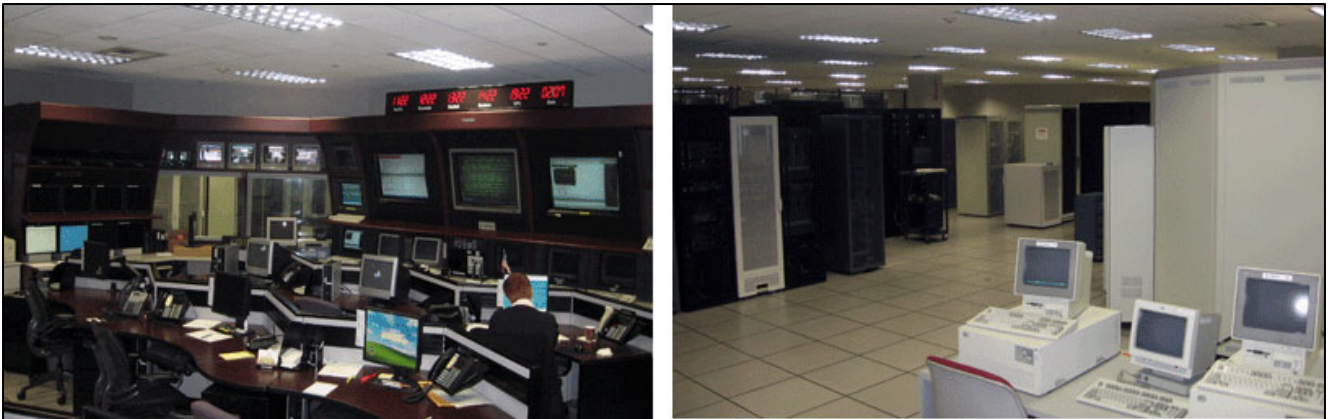
The Orange County Data Center (OCDC) was rated as a Tier III facility, more reliable than all Agency Data Centers rated as Tier II facilities.
